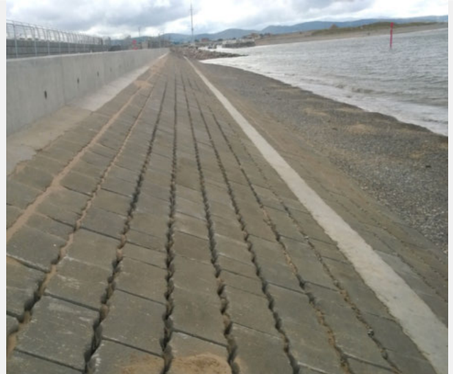
Linked concrete blocking surrounded by C40 concrete containing 4 kg Durus S400. Protecting the land from coastal attack and erosion.
