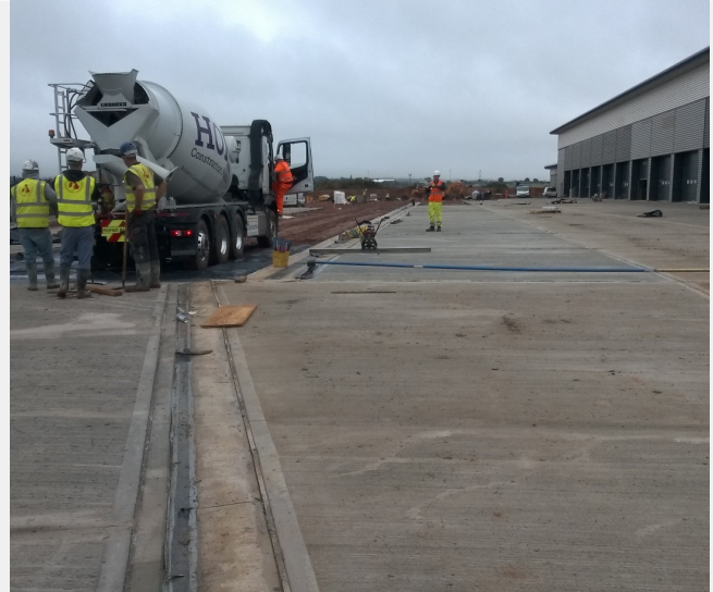
As the reinforcement is dosed into the concrete during batching, the mixer truck can discharge directly into the formwork.
