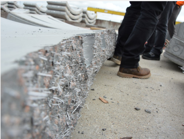
Fullscale trial elements were broken to ensure consistent dispersion of Durus S500 macro synthetic fibres throughout the whole volume of the units.
