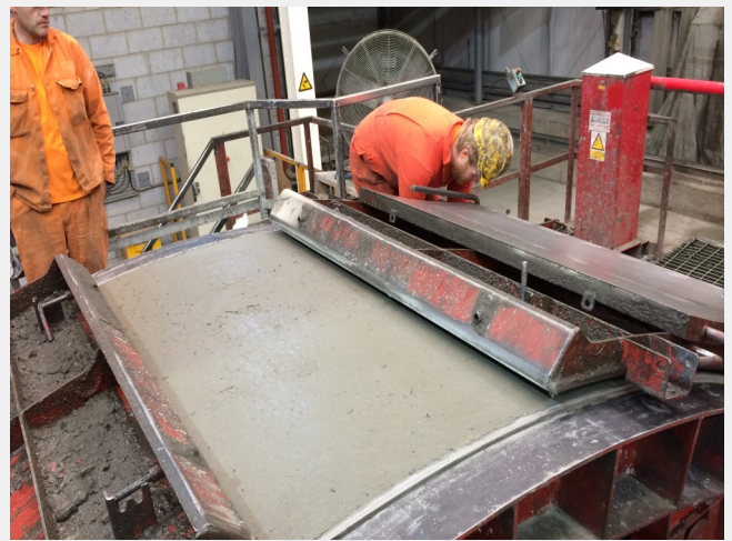
During trials, opening of segment moulds confirmed a high quality surface finish of elements containing Durus S500.
