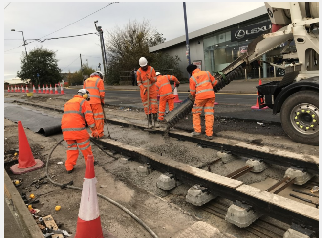
Midland Metro project, UK, during installation of Durus EasyFinish fibre reinforced concrete
