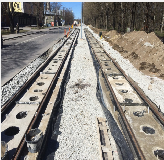
Tallinn Tramline project. When completed, the tram route will be planted with grass to provide a 'green' route around the city.
