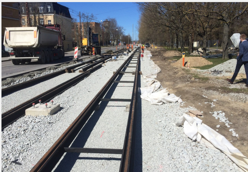
Prior to installation of the Durus EasyFinish MFRC Track Slab - Tallinn, Lithuania
