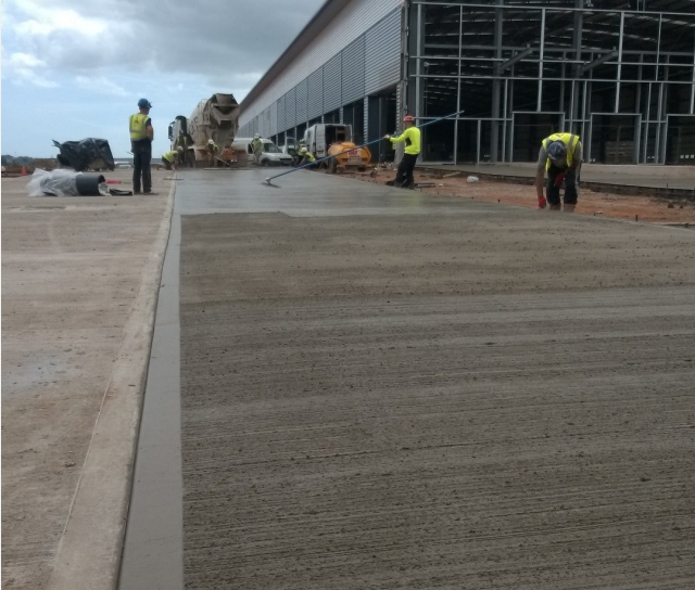
By eliminating steel mesh, large areas can be poured/finished, with saw cut contraction joints being made the following day.
