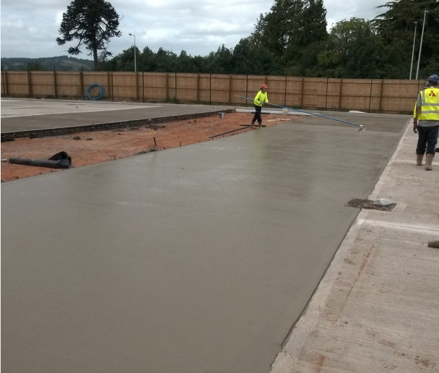
By eliminating steel mesh, large areas can be poured, with saw cut contraction joints being made the following day.
